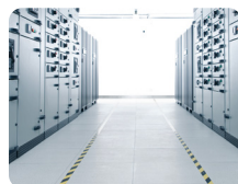
Security warning equipment
